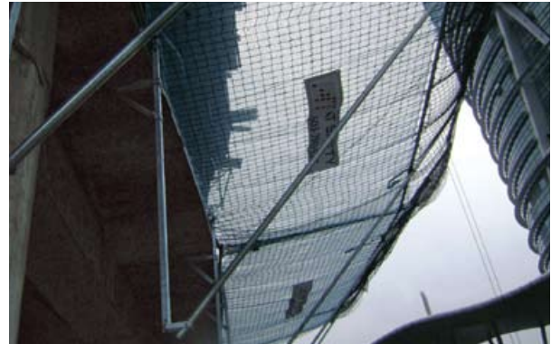
Fall Arrest Safety Nets prevent falling debris from causing injury to people underneath
