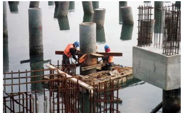
Proper installation of brackets for piles in accordance with quality procedures at our berth expansion project, Kuantan Port
