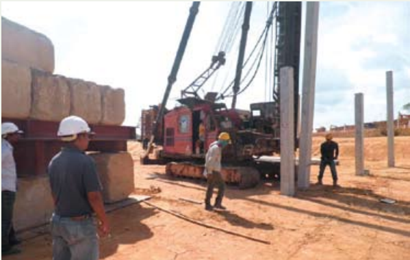
Use of custom made guide to pitch square piles in the correct position at our Perkeso Rehabilitation Centre Project, Malacca
