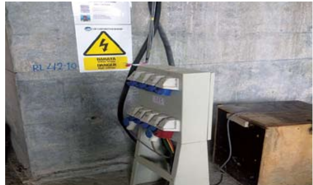
Industrial DB board installed at construction sites to prevent short circuits
