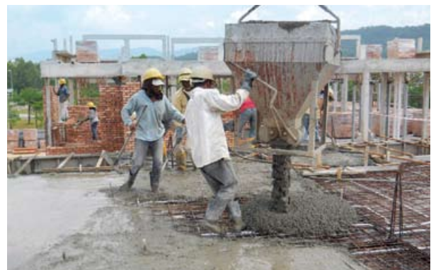
Proper apparatus are used to maintain the quality of our concrete and brickworks at our Aviva Green Project, Seremban 2
