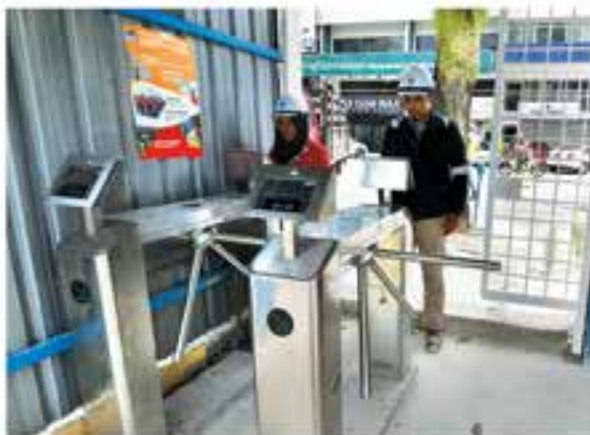
Controlled site access and egress with turnstile and biometric system
