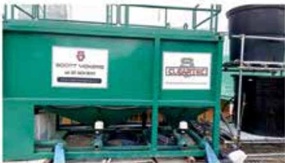
Wastewater treatment system implemented at the construction site to ensure water quality complies with the stipulated limits
