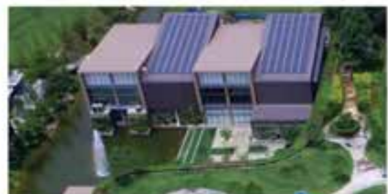
PV solar panels installed on the sales gallery building roof
