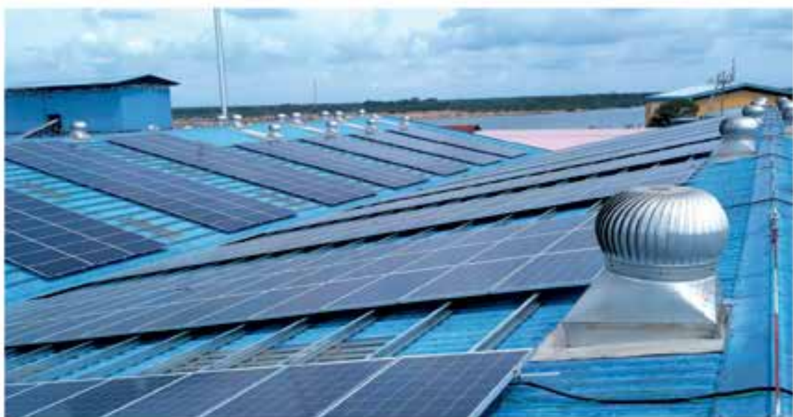
Rooftop solar PV system at Lumut factory
