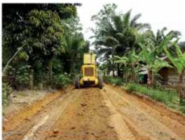
Road maintenance for better accessibility for neighbouring communities in Lampung estate, Indonesia
